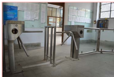
RFID access control gate
